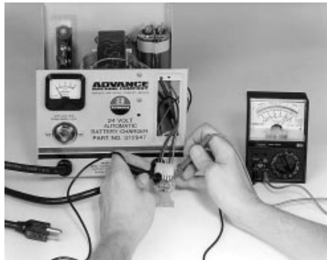
FIGURE 3. Measure battery system voltage at the test kit pads.
